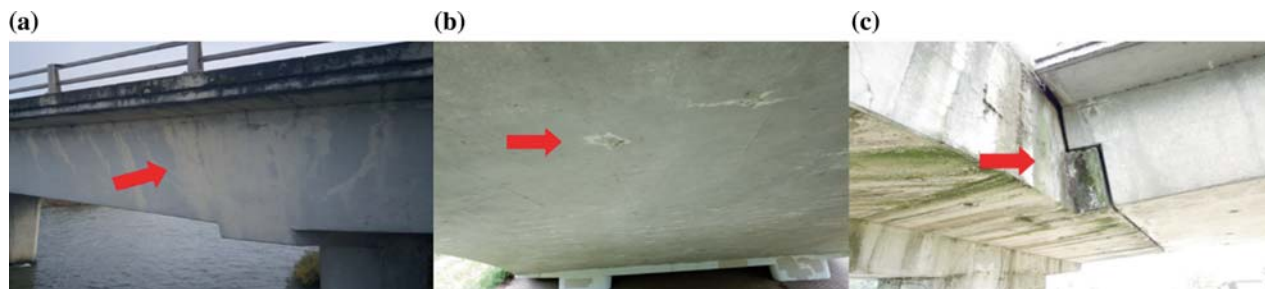
Fig. 74.3 Sample images of defects: a cracking with efflorescence on the side of the box b spalling area underside the box c rust staining on the concrete column
