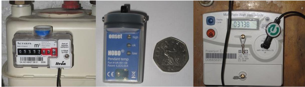
Figure 3: From left to right – gas meter fitted with pulse module, hobo pendant sensor used for temperature monitoring and electricity meter fitted with LED pulse detector.
