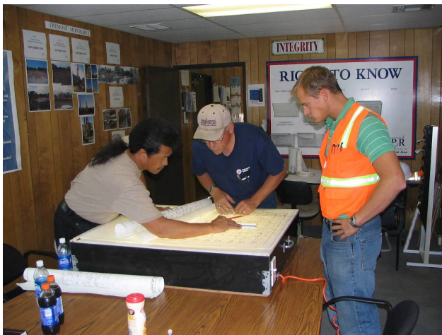
Figure 2. MEP coordination session at the Palo Alto Medical Foundation Project in Fremont, CA, USA using the SCOP. Drawings representing different trades are overlaid on a light table to detect clashes between the MEP systems. Image courtesy DPR Construction, Inc., CA, USA.
