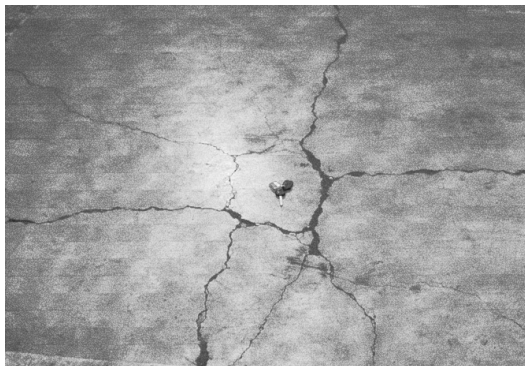
Figure 9. Pattern of cracking around a local hard spot [29]
