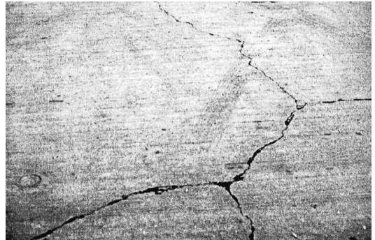
Figure 8. In some bays, the cracks quartering the bay are connected by a short 45 degree crack [27]
